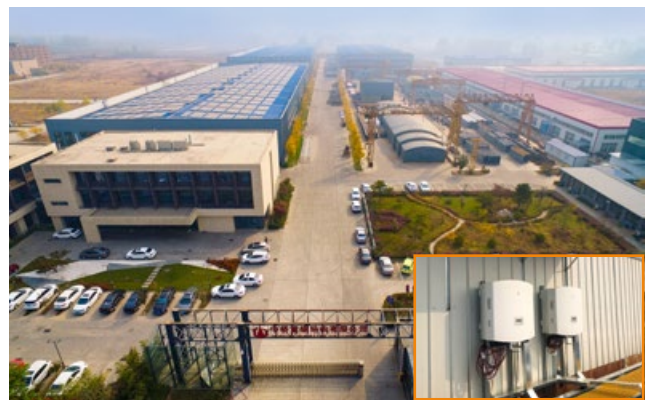
Hebei ZQ Steel 1.5MW
