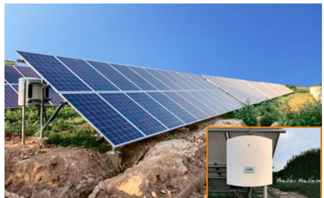
Hebei Qinghuangdao poverty alleviation PV Plant 5MW
