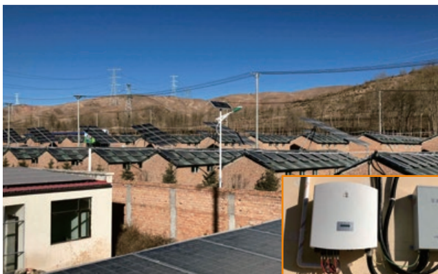
Qinghai HuzhuBanyan poverty alleviation PV Plant 2MW
