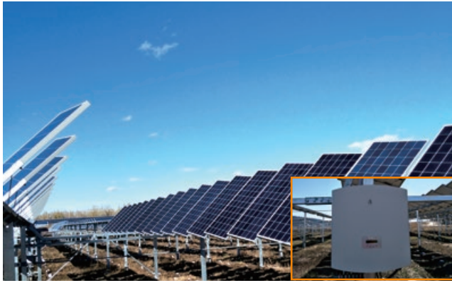
Hebei Zhangbei Agricultural-photovoltaic hybrid PV plant 50MW
