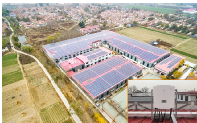
Shandong YUELONG 3.5MW
