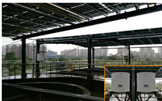
Hunan Yongzhou dao county water plant 800kW
