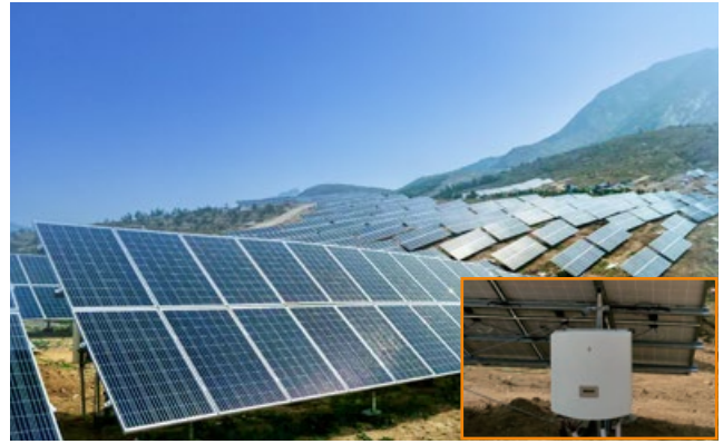
Liaoning Yingkou Jiuzhai PV plant 20MW
