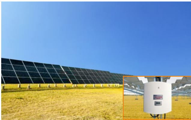
Huaneng Yimin surface mine PV plant 20MW
