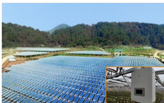
Zhejiang Dajie Agricultural-photovoltaic hybrid PV plant 3MW
