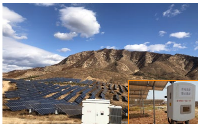
Liaoning Gaizhou Jiuzhai PV plant 20MW
