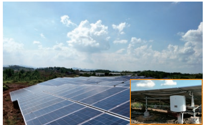
Jiangxi Ganzhou PV Plant 3.5MW
