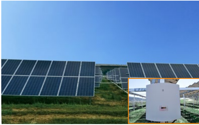
Hebei Zhangjiakou poverty alleviation PV Plant 5.1MW
