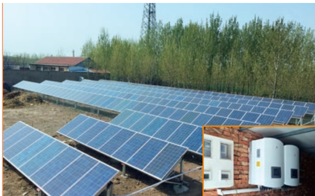
Shandong Leling poverty alleviation PV Plant 50kW
