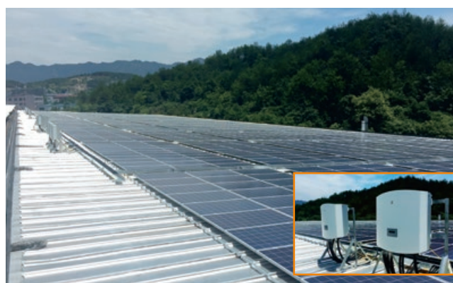
Hainan JiuLongGlass 1.7MW
