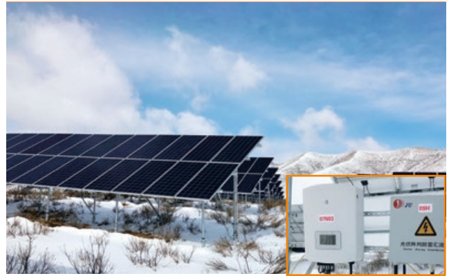
Shanxi Guangling PV plant 1.47MW
